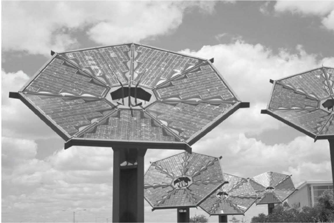
Figure 1-3 Solar collector field. 1
